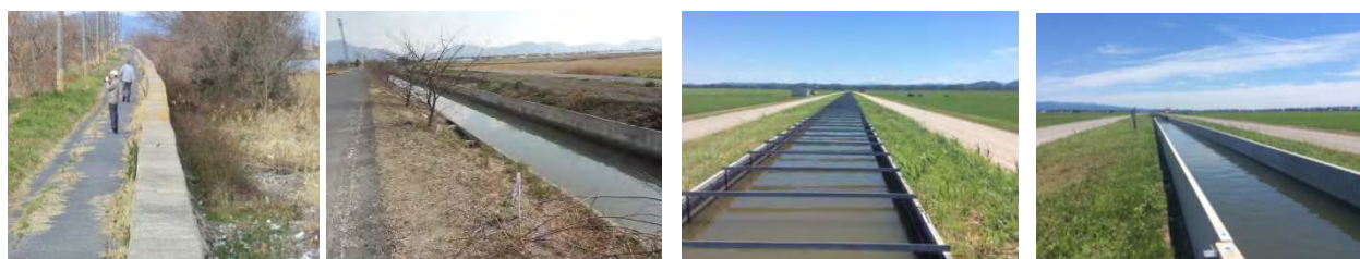
(a. 不陸のある海岸堤防) (b. 矢板に損傷のある開水路) (c. コルゲート開水路：A地区) (d. 試験化施工開水路：F地区)
