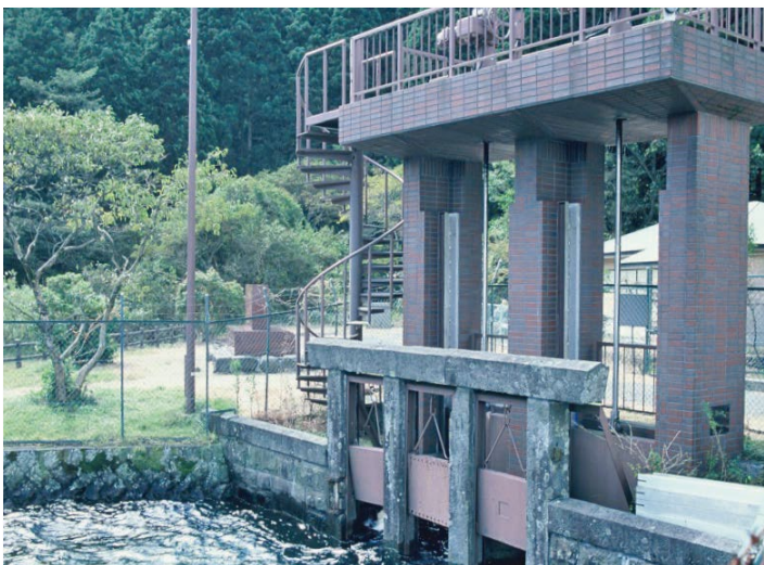
Fukarayousui Watergate (the intake at Lake Ashi)
