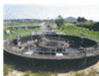
Neribeya diversion station
