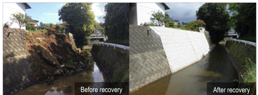
Damaged canal by the Kumamoto earthquake 2016 (Uwaide Canal)
