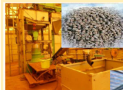
Pelletizing facilities Pellet compost (upper right)
