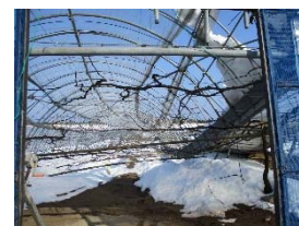
Damaged grape greenhouse (Tottori)
