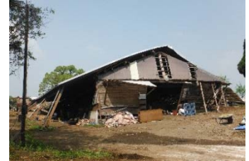
Collapsed animal house barn
