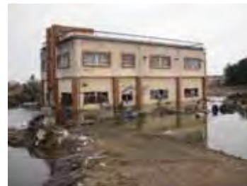
A drainage pumping station crippled by tsunami waves (Natori City, Miyagi Prefecture)
