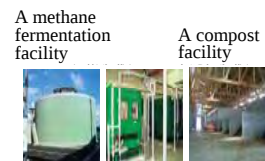
Biomass conversion facilities (Yamaga City, Kumamoto Prefecture)
